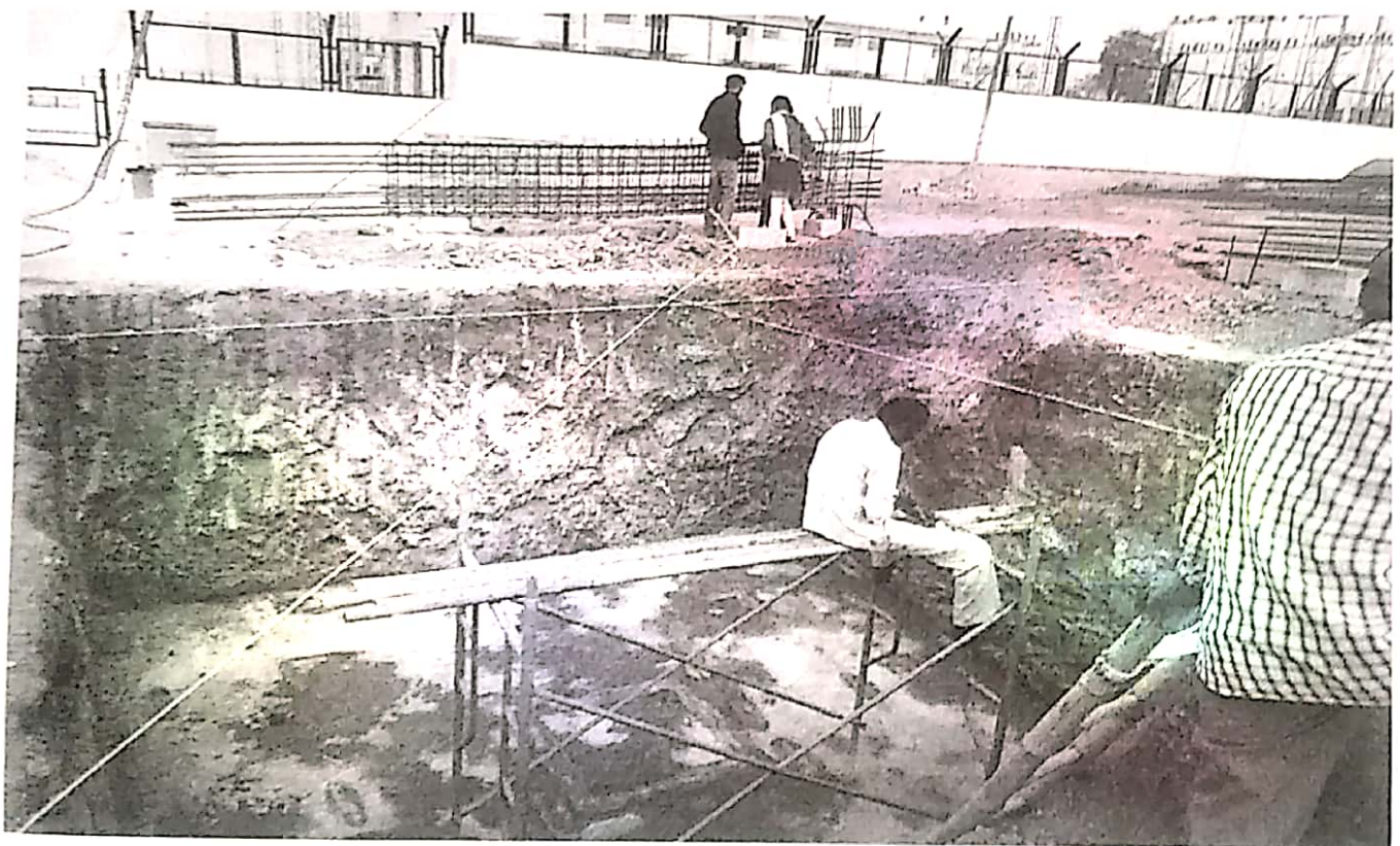
Locating and transferring the Centre Point of Column with the help of Plumb Bob from the Grid line marked with the suspended wire.
